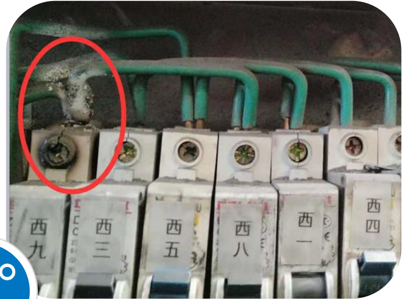
Risk of the power distribution cabinet lines
